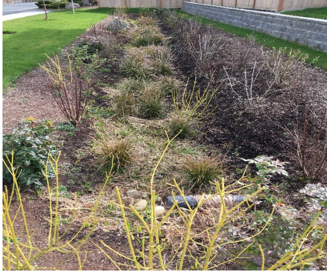
Bio-retention facility recently installed in a newer housing development.
