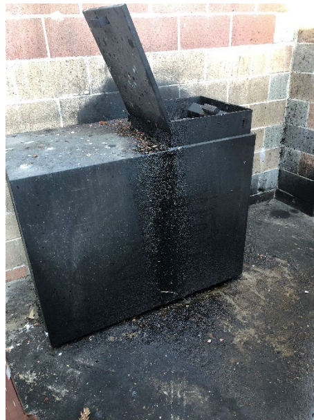
City staff reported a grease/food waste spill and open container at a restaurant during the initial dumpster outreach campaign visit.
