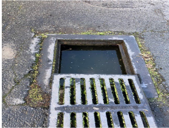
Between annual facility inspections and the GIS Technicians continued mapping of the MS4, issues such as these are becoming less and less prevalent.
